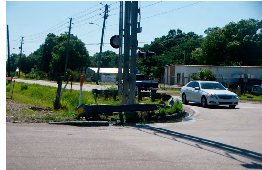
Damaged guardrail caused by turning trucks at the intersection of Wabash Avenue and Olive Street in Lakeland
